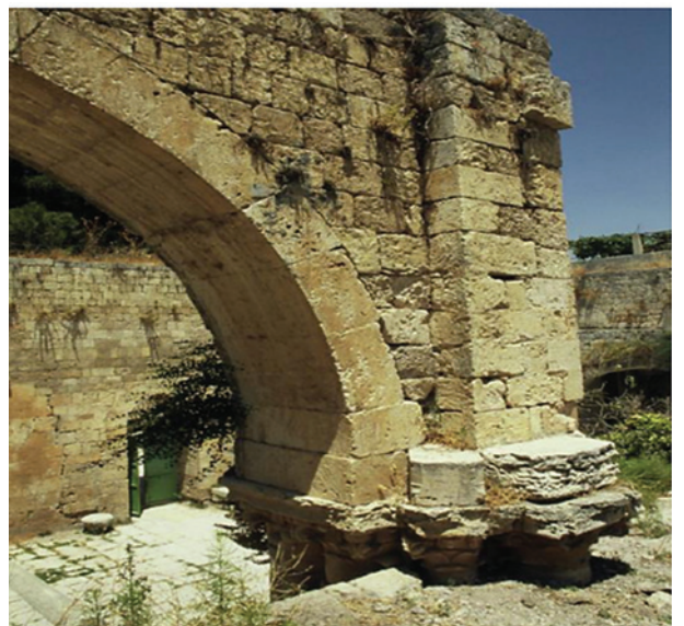
PLATE 25.16 Combined pillars and capitals at the church of St. John in Sebaste. PHOTOGRAPH BY MOSHE MILNER.
